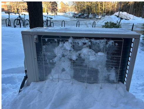
Figure 13: Ice and frost build up on the outdoor ASHP coils after a winter snow storm
