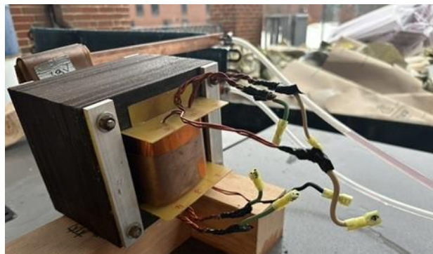
Figure 17: Transformer with quick slide connectors attached to all six primary leads to allow for easy and quick changes in secondary voltage outputs
