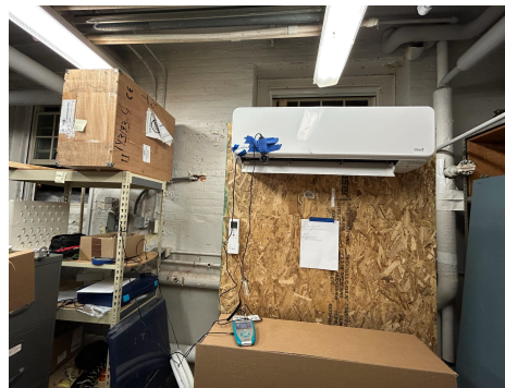
Figure 7: The indoor set up of the AHU featuring the ambient temperature sensor 75 cm away, the outlet anemometer and outlet temperature directly at the outlet fan of the unit, additionally showing the LabQuest used to store and log the data
